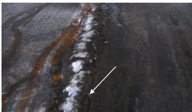
Figure 1. Crack in the weld zone of the welded joint
